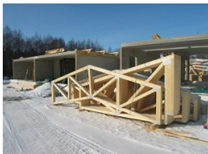
Figure 5.3.2: The members of these trusses all lie in a single plane. These roof trusses are an example of a plane truss. Image by Riisipuuro CC-BY-SA 3.0.
