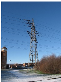
Figure 5.3.5: The power line tower also does not lie in a single plane and is therefore a space truss. Image by Anders Lagerås CC-BY-SA 2.5.
