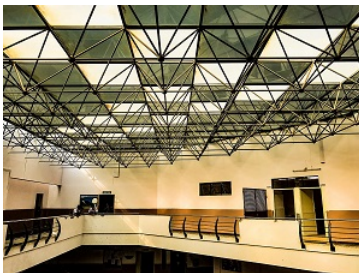
Figure 5.3.4: This roof supporting truss does not lie in a single plane. This is an example of a space truss. Image by IM3847 CC-BY-SA 4.0.
